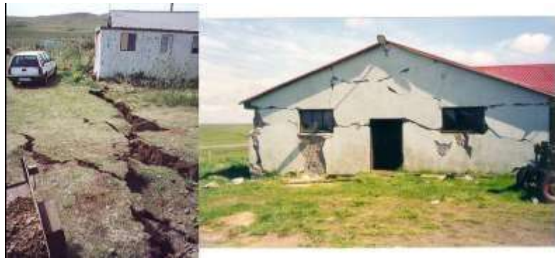
Fig1. Damage of building because of earthquake
