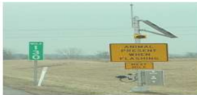
Fig. 2: The system arrangement on pole used on highway
