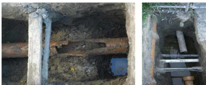
Figure : Broken pipes in earthenware laterals and difficulty of applying open-cut method. (Images by author of paper)
