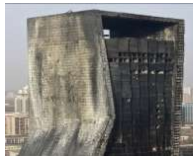
Fig 1.2: Fire Damaged Building
