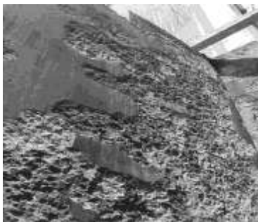
Fig.1.1: Fire Damaged Concrete Surface
