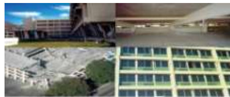
Fig.2 Damages of various buildings
