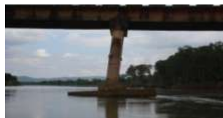
Fig.3 Damage of bridge pier
